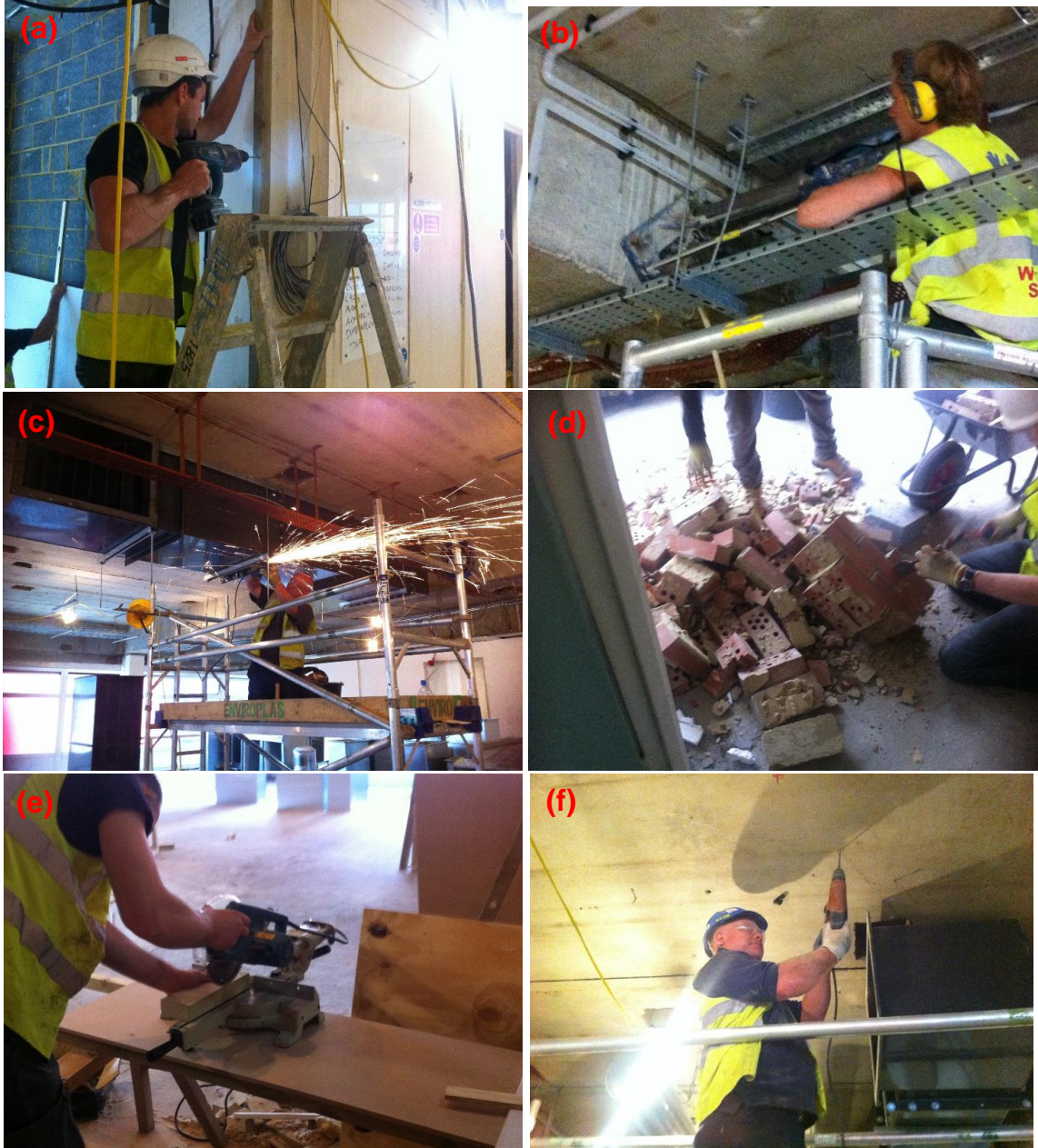
Figure 5.2: Number of typical activities involved in refurbishment works including (a) drilling of wood, (b) drilling of concrete slab, (c) cutting, (d) hammering, (e) sanding and (f) ceiling drilling activities.
